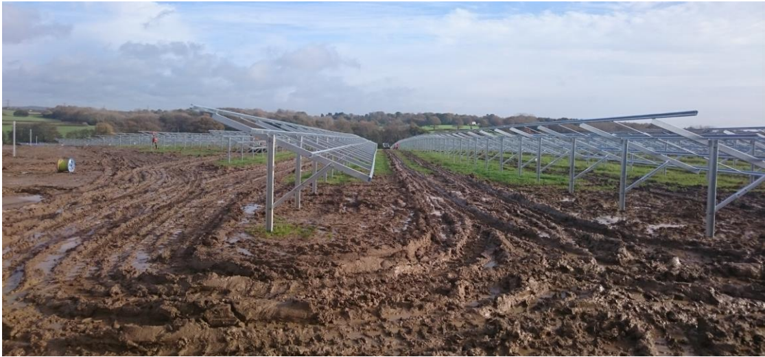
Inserts 35 and 36: Winter Installation (2015) and Operational Site (2022)
